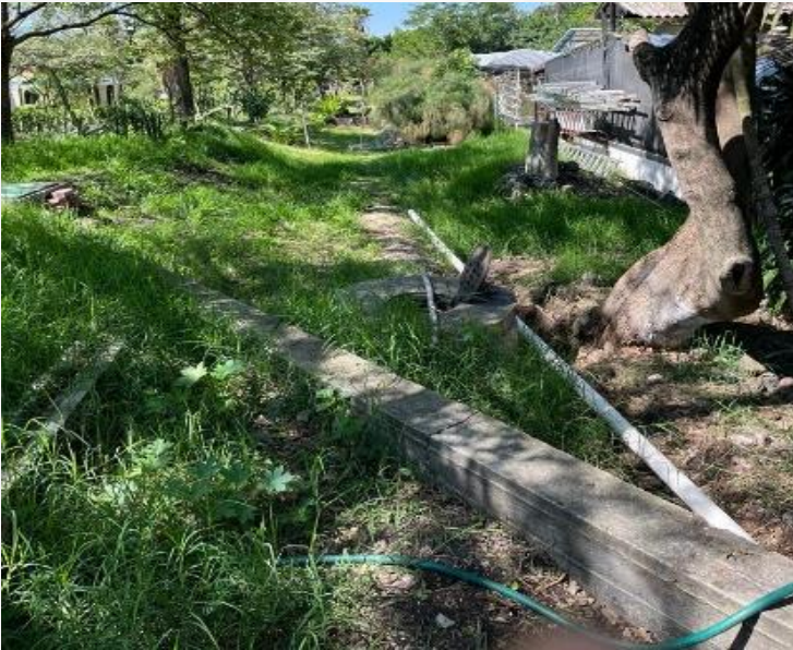
4-inch conduit to rain garden
