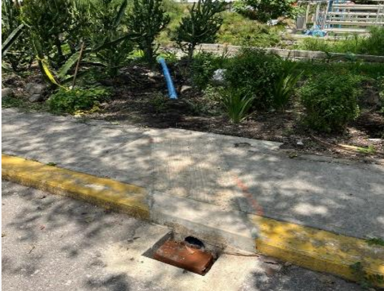
Grate and conduit to rain garden
